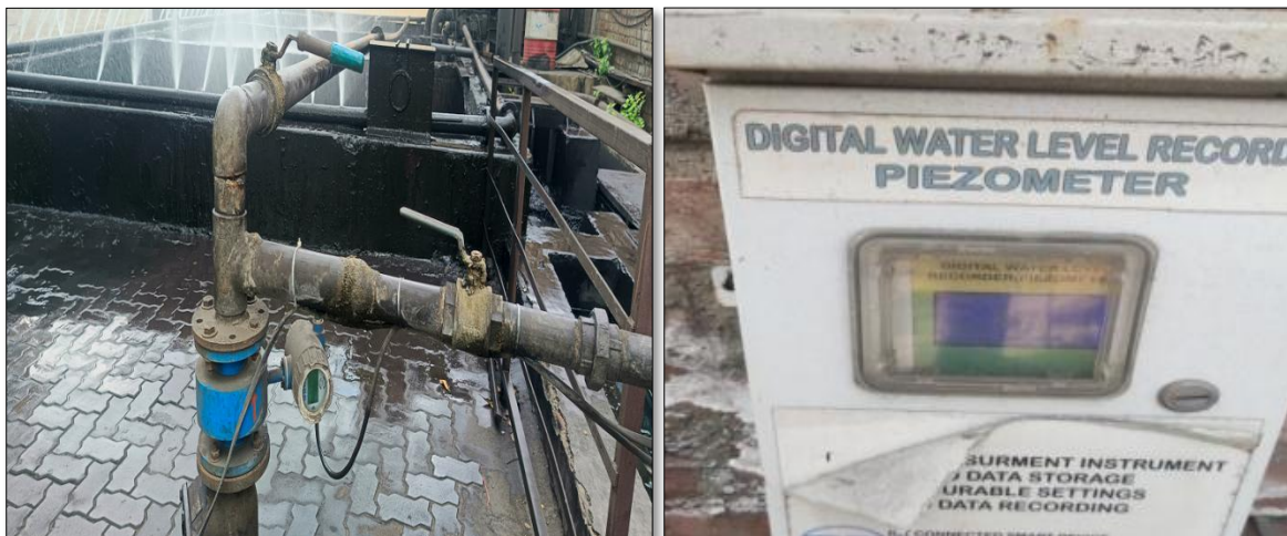
Figure 1-2 Water Flow Metre & Piezometer
