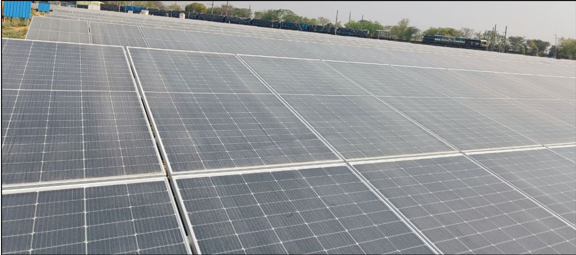
5MWp Solar Plant at J.K. Cement work- Nimbahera, Rajasthan
