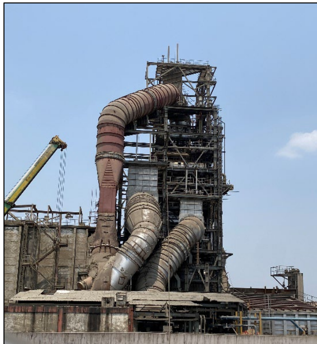
Waste heat recovery system of Muddapur
