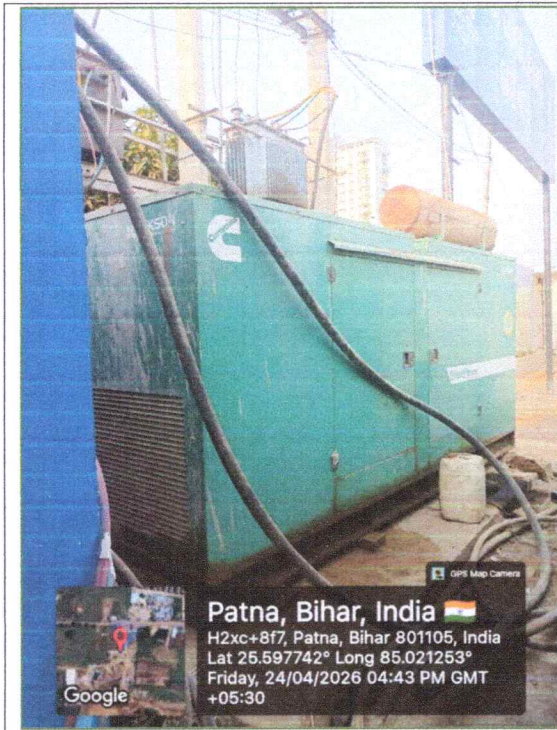
DG Sets with acoustic enclosures
