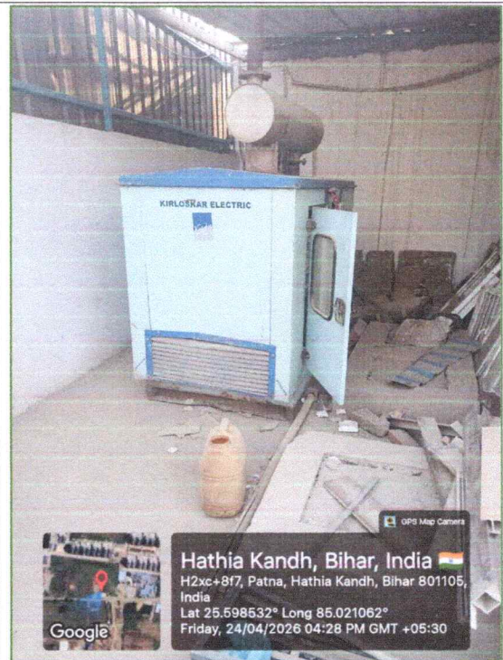
DG Sets with acoustic enclosures
